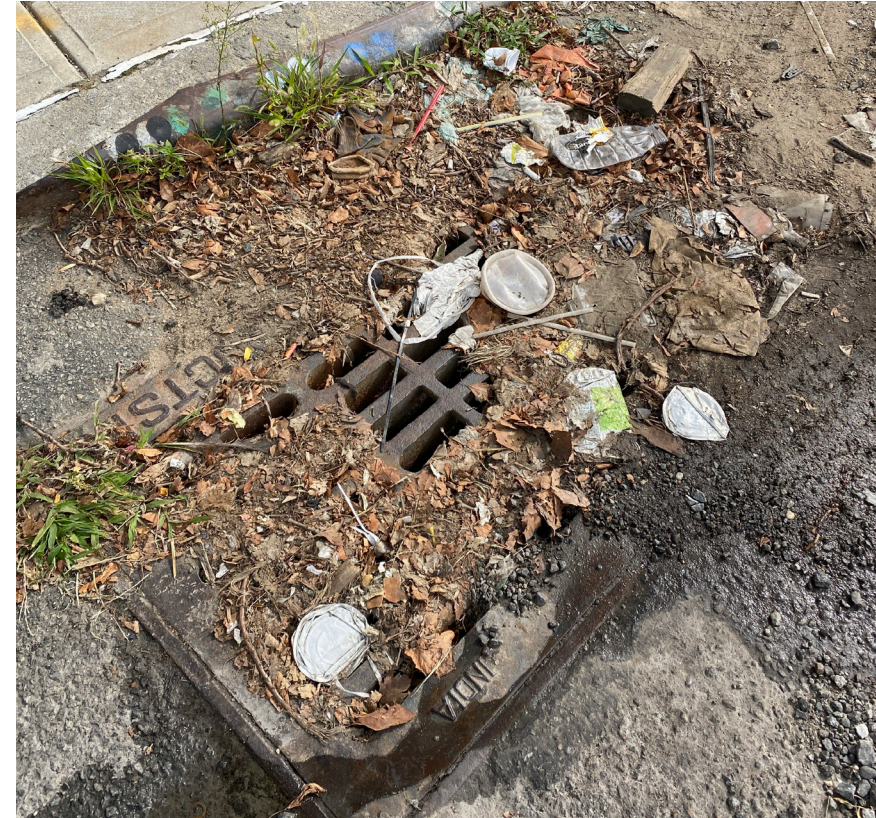
Clogged Catch Basin
